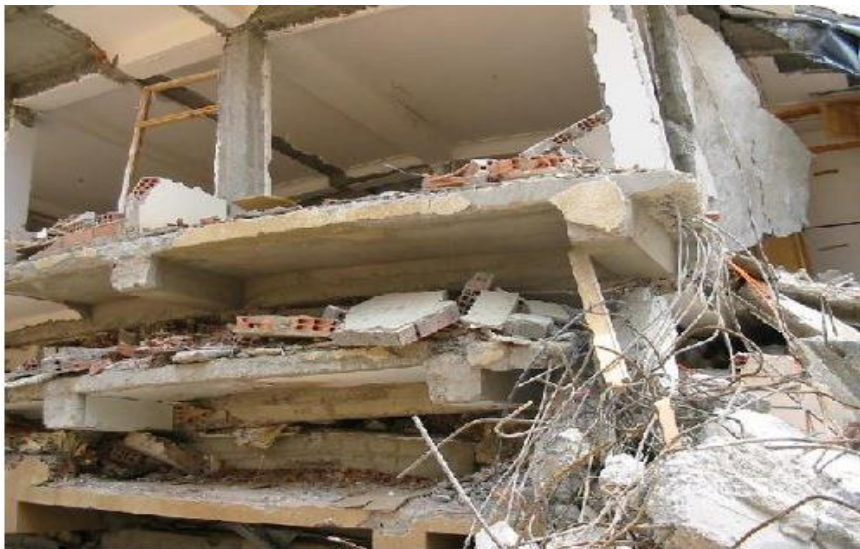
Figure I.2 : Effondrement total de la structure. [5]
