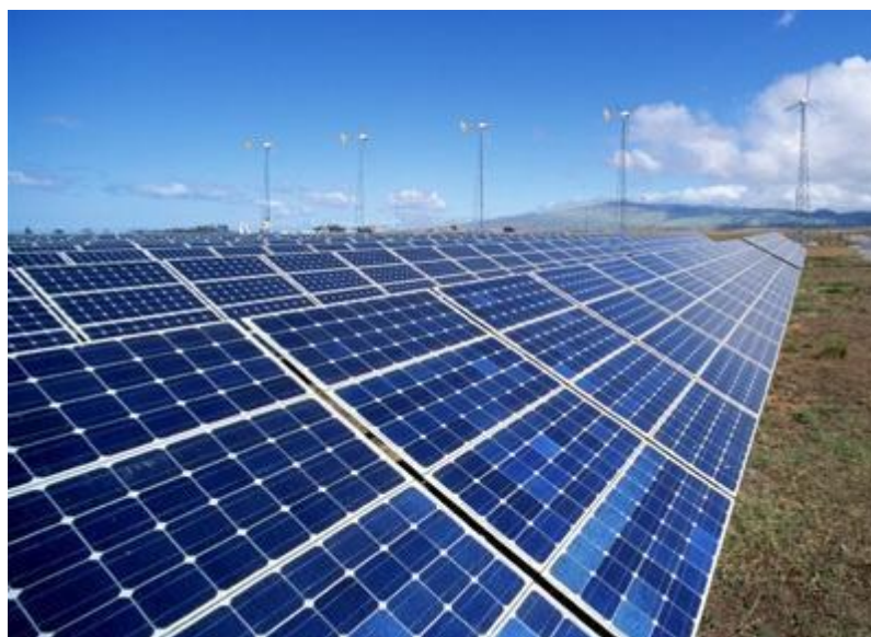
Figure I.6 Panneaux Solaires Photovoltaïques.
