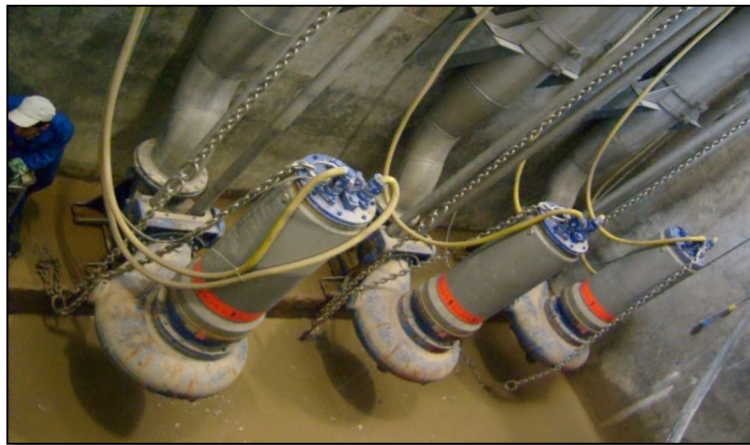
Figure III.2 : Station de relevage des eaux brutes
