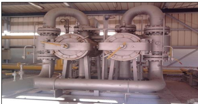
Figure II.4 : Skid de filtration.
