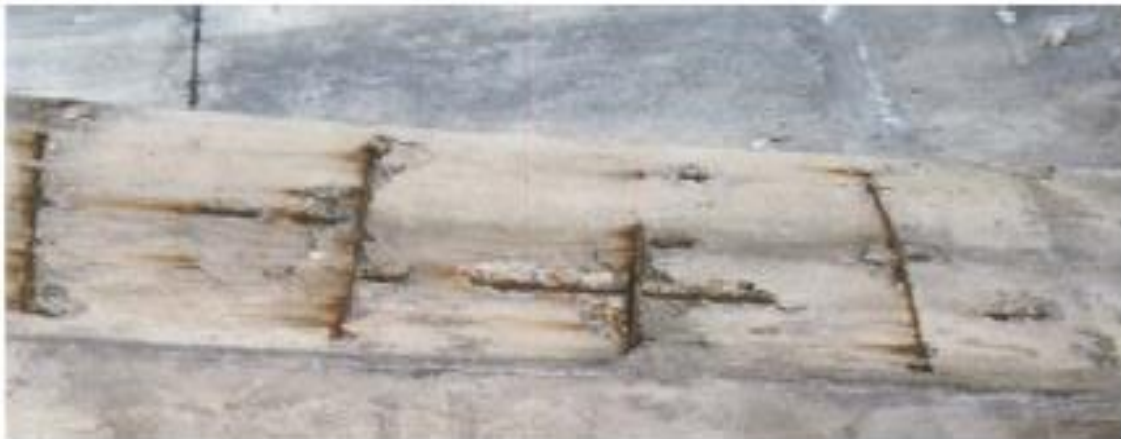
Figure I. 2. Corrosion des armatures
