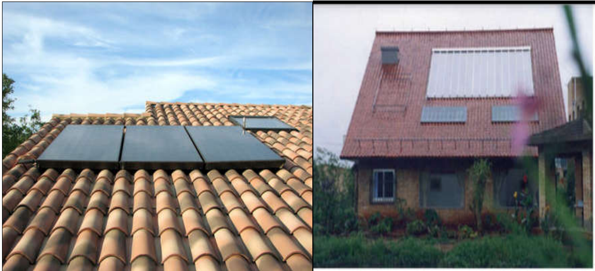
FIGURE III.3: south-roof partially covered by solar collectors [4].
