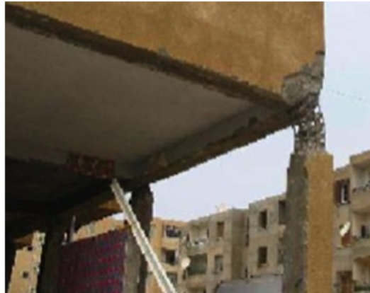
FIGURE 2.21 – Plastification des poteaux
