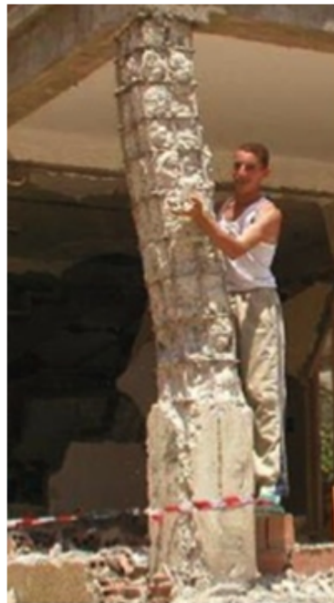
FIGURE 2.22 – Plastification des poteaux
