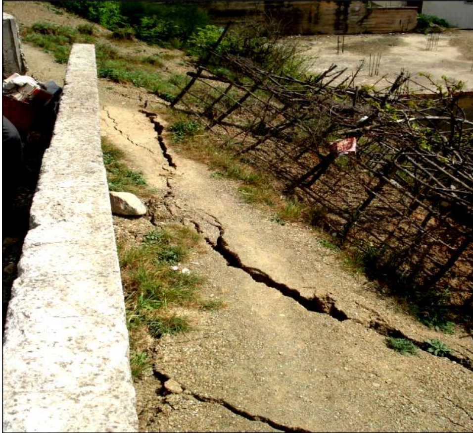
Figure I.3: Photo montrant les fissures de traction
