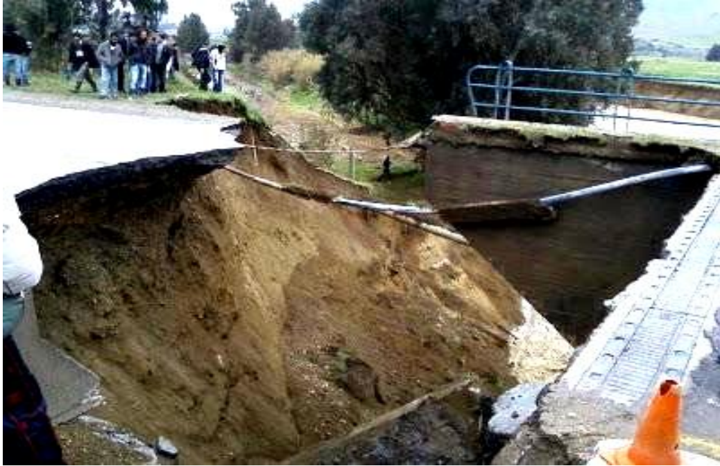
Figure II.11: Glissement Tala Méhalef TIZI OUZOU
