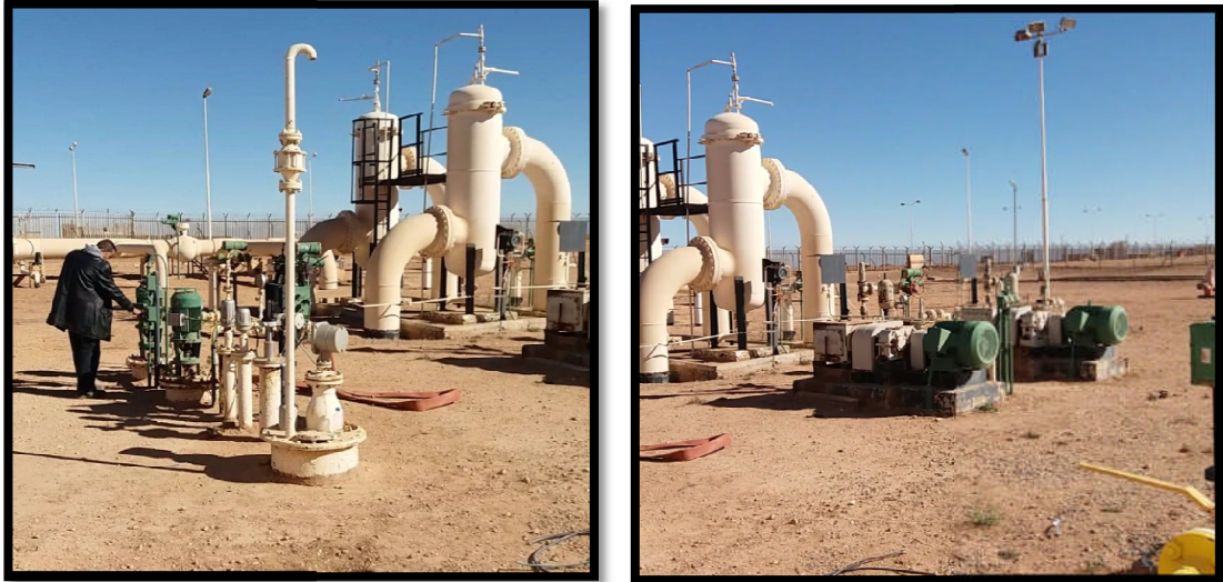
Figure III-17 Pomperiegavage (refoul. 4 bar) et transfert(refoul.38 bar)
