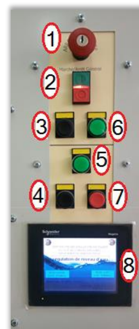
Figure II.2 Poste de control
