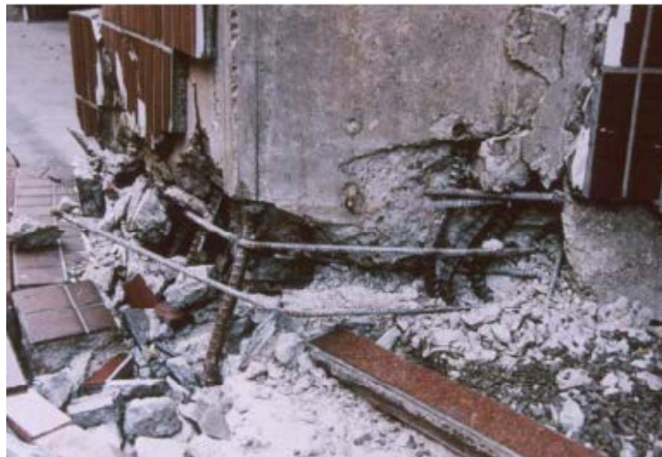
Figure II.6 : endommagement au pied du poteau
