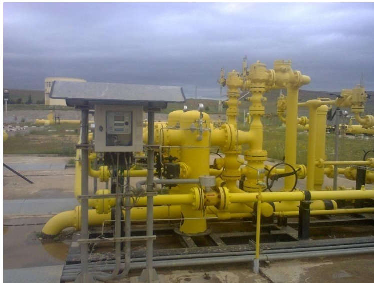
Figure 5 : Skid filtration de la station SC4 Nador.
