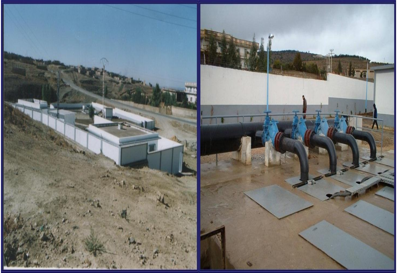
Figure II.3: station de relevage de Tiaret
