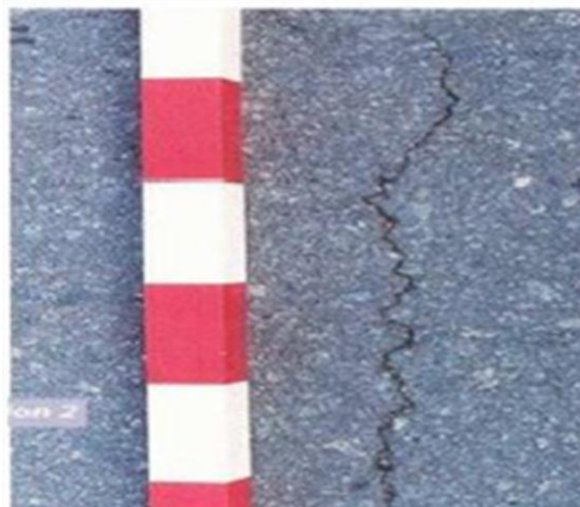
Fig.(I.22) Fissuration transversale : fissure franche et perceptible [LCPC, 1998][7]
