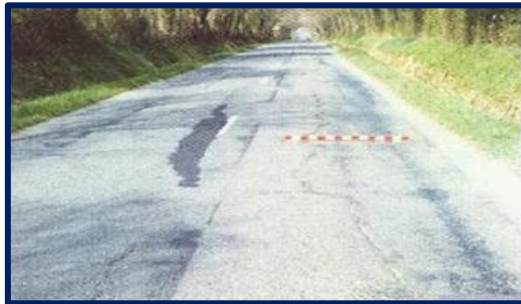
Fig.(I.25) Fissure d'adaptation [LCPC, 1998][7]
