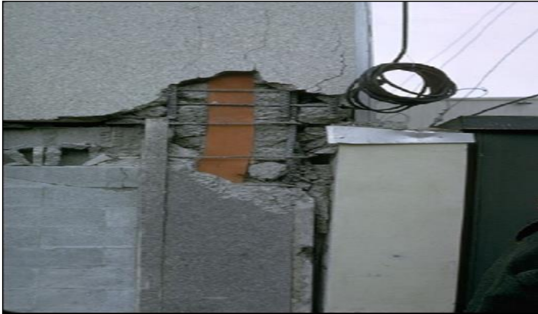
Figure 1.13 : Joint parasismique insuffisant
